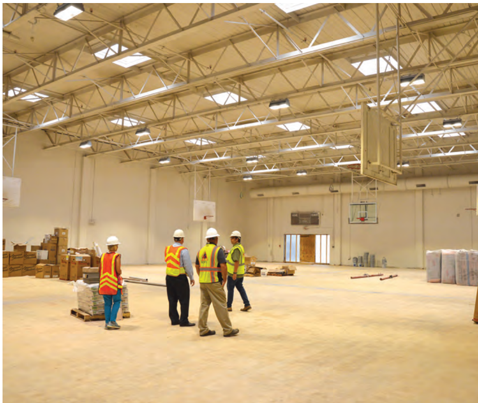
The gymnasium at W.B. Wicker Elementary School isn't new, but the floor and goals will be. One of the final touches to the refurbished school will be the flooring in the gym, which might be one of the few things not quite ready for use when school starts later this month, according to school officials.
