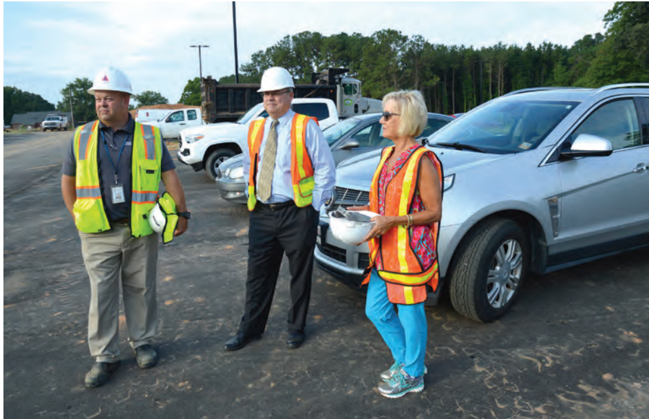
Superintendent Andy Bryan, flanked by District Maintenance Director Chris McNeil and LCS Public Information Officer Sharon Spence, prepares for a tour of the construction site of W.B. Wicker Elementary School in mid July, just over a month before the school's opening.
