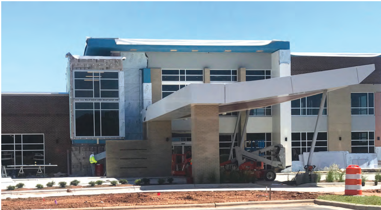
The new terminal at the Raleigh Executive Jetport in northern Lee County was nearing completion as of the publication of this paper, with airport leaders are saying they expected the project to be “substantially completed” some time during the first week of September, with move-in coming later in the month. The $4 million terminal building is part of a facility that generates $61 million in annual economic activity. Plans will be announced soon for events to mark the opening, likely in October. Photo by Gordon Anderson.
