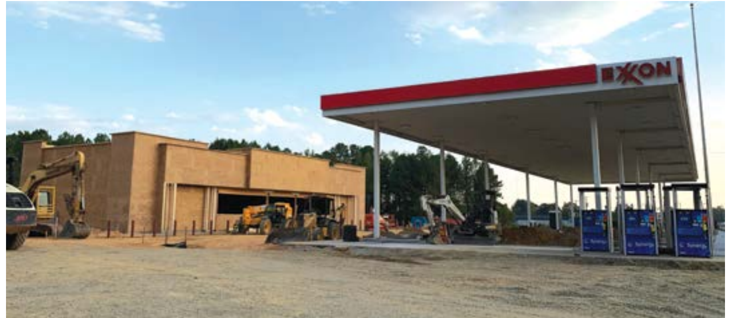
PROGRESS AT NEW TRAMWAY GAS STATION | While we haven't heard of an opening date, progress is visible on the 5,000 square foot Circle K "mega store" on U.S. 1 in Tramway. Work began in early August.
